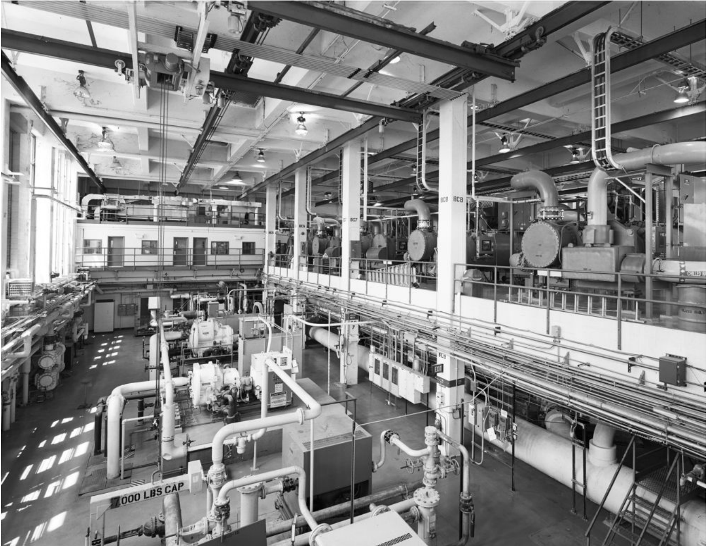
Kansas City Plant power house, 2013 (Historic American Engineering Record, U.S. Department of the Interior/Richard Welnowski)
