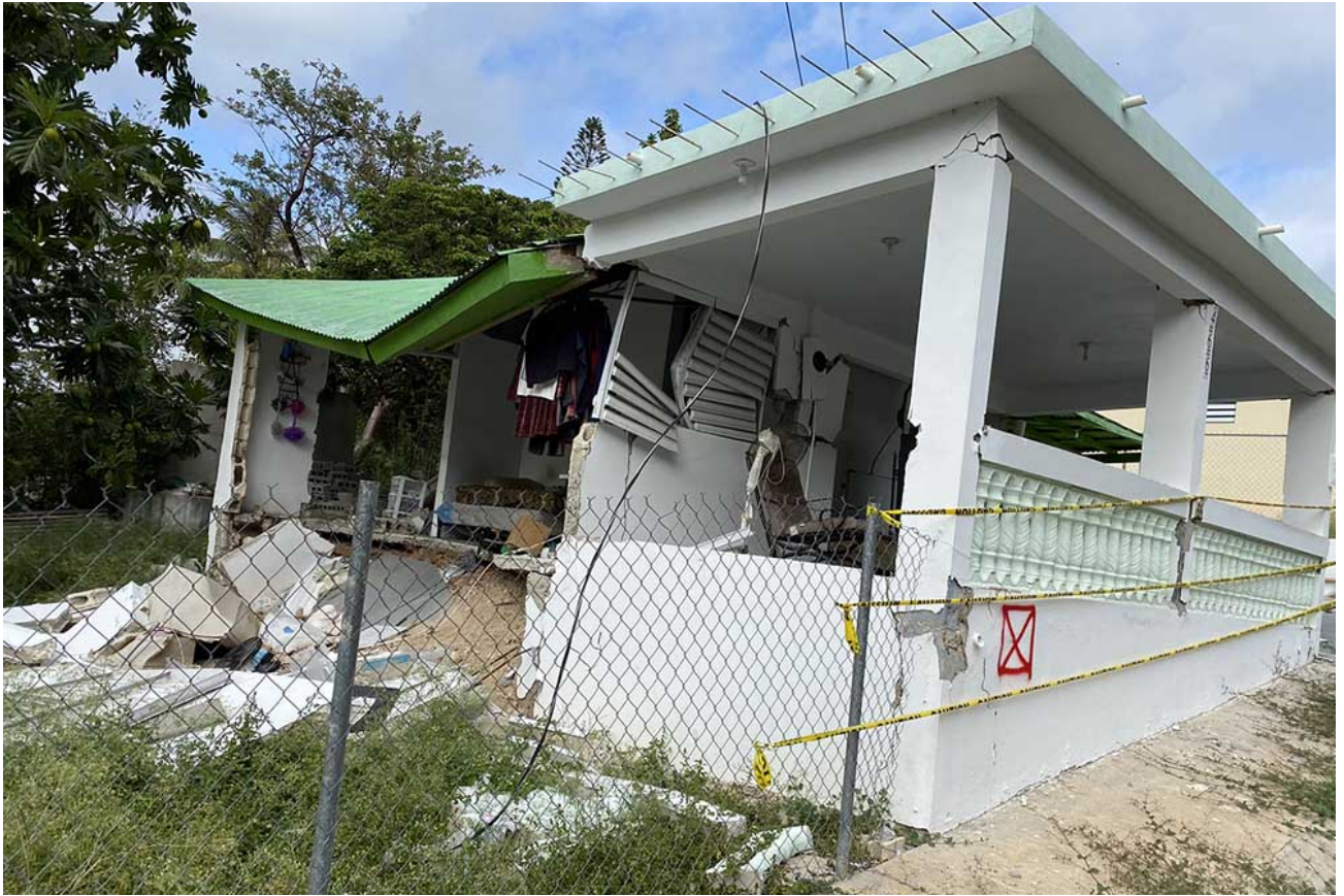
Home after home in this neighborhood in Guánica is designated red, meaning it's unsafe to enter. (GSR photo / Soli Salgado)
