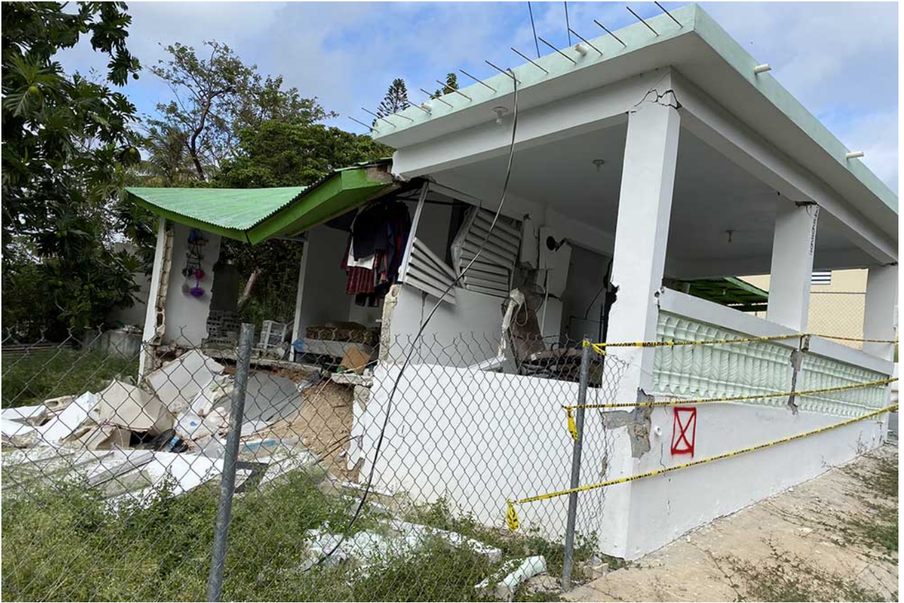
Home after home in this neighborhood in Guánica is designated red, meaning it's unsafe to enter. (GSR photo / Soli Salgado)
