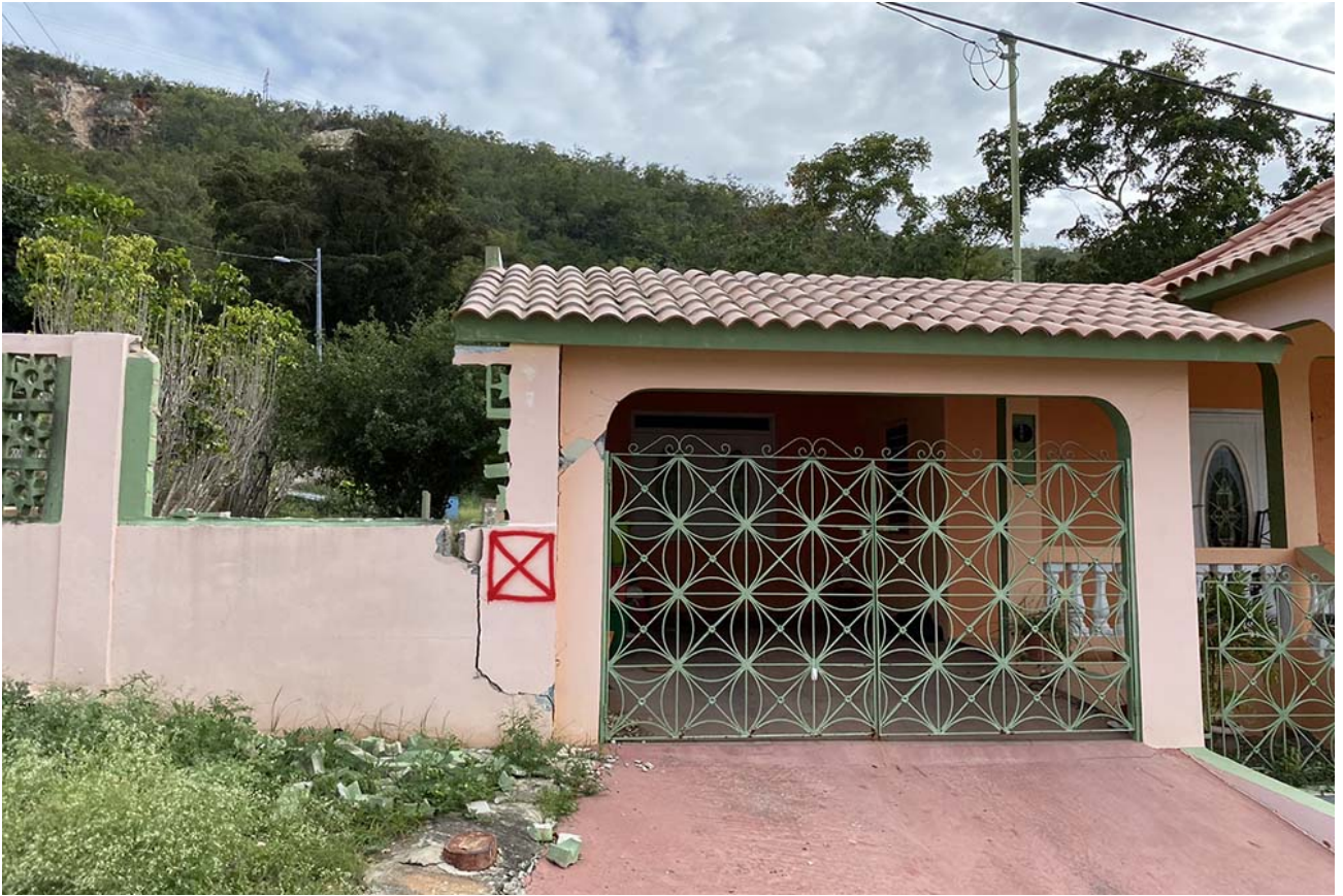
Home after home in this neighborhood in Guánica is designated red, meaning it's unsafe to enter. (GSR photo / Soli Salgado)
