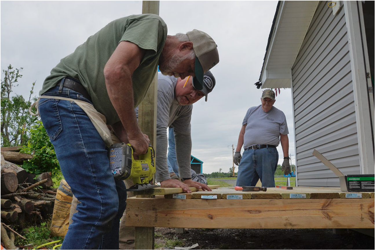
From left: Jude Leake, Ed Mattingly and Rick Wagoner build a new porch on a home May 23, more than six months after a tornado badly damaged the home in Mayfield, Kentucky. (GSR photo/Dan Stockman)
