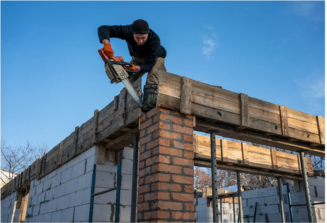
Despite the tragedy of the massacre of civilians in Bucha, Ukraine, as well as the destruction of property, families are reconstructing their homes — and, by inference, rebuilding their lives. (GSR photo/Chris Herlinger)
